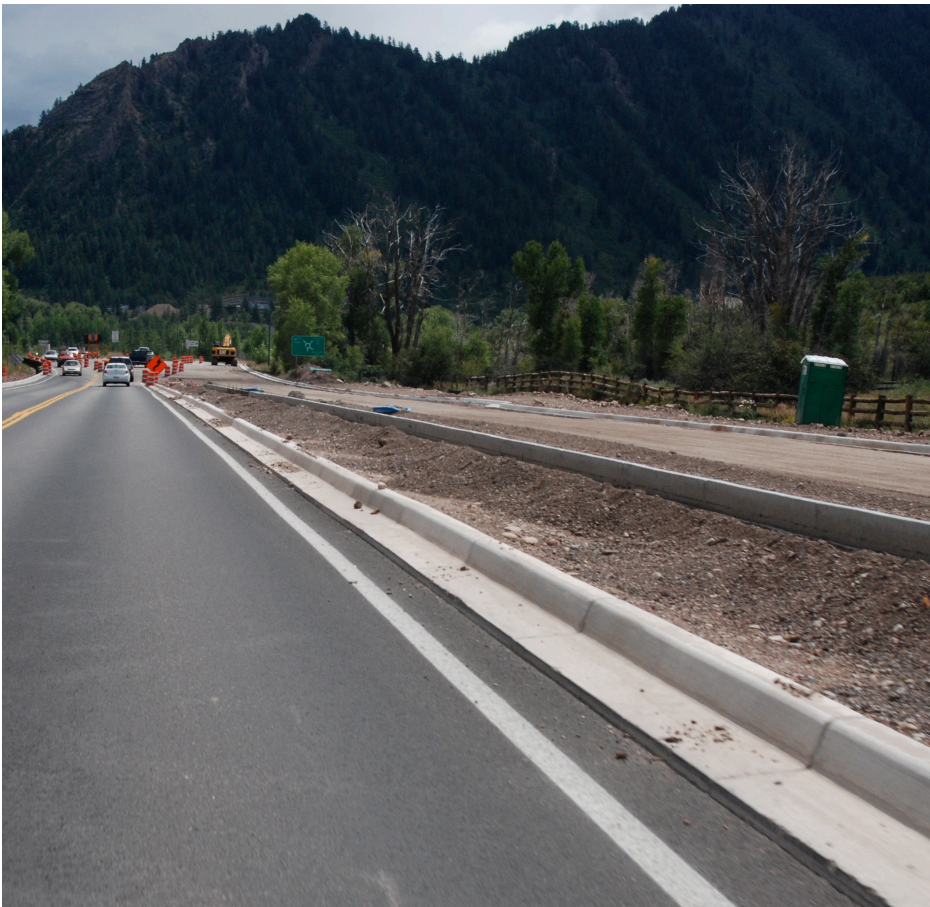
Construction of the bus lanes from the airport to the roundabout in 2008.
